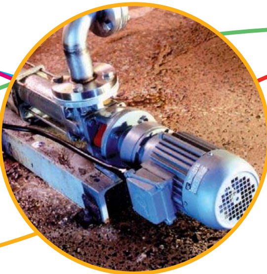
Transfer of industrial detergents
